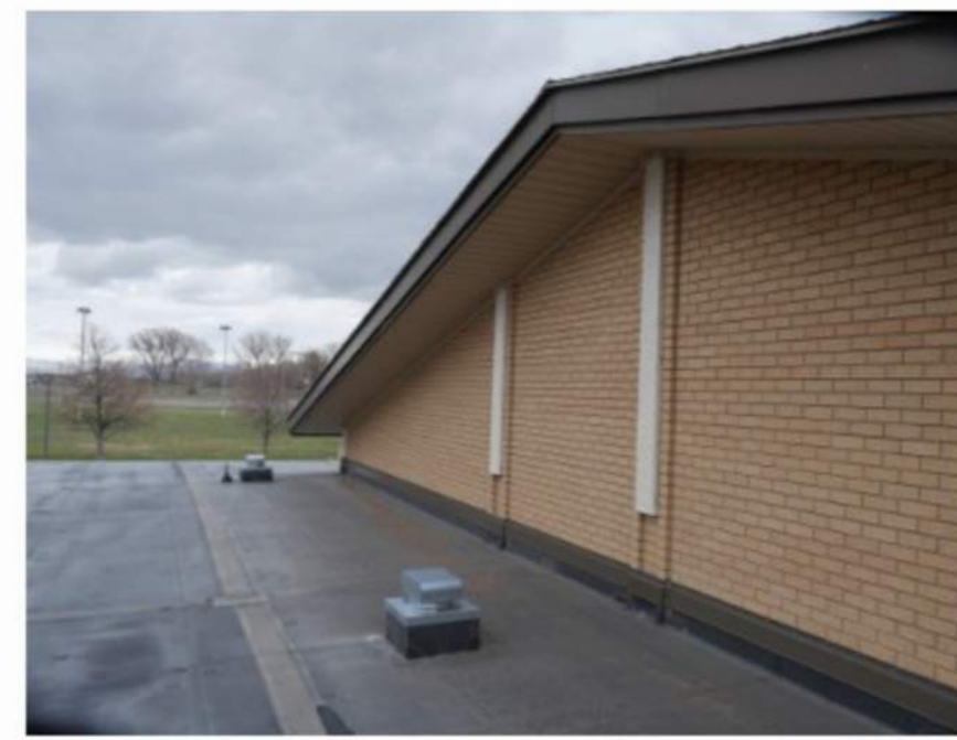
Remove flashings and counterflashings. Install new to match color of existing fascia after installation of new roofing material. Protect heat cable from damage and re-install after new roofing is complete.
