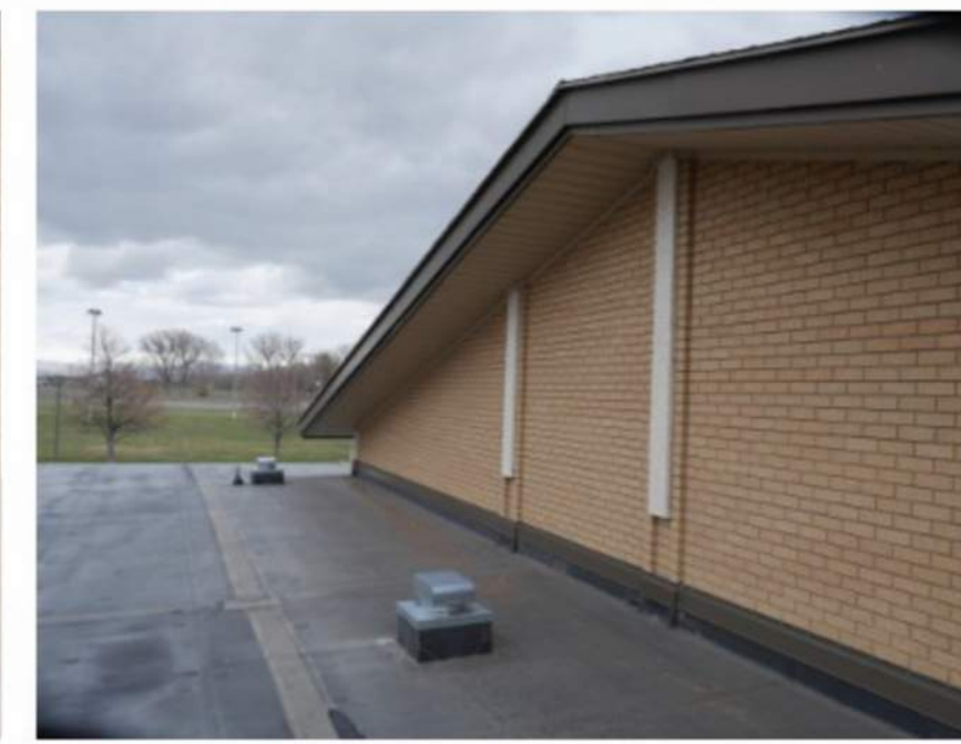
Remove flashings and counterflashings. Install new to match color of existing fascia after installation of new roofing material. Protect heat cable from damage and re-install after new roofing is complete.
