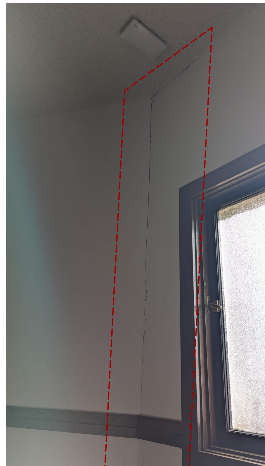
A2 CRACK AT UPPER STAIR WALL
