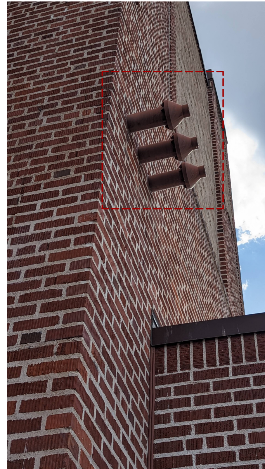
C3 MECHANICAL VENTS
