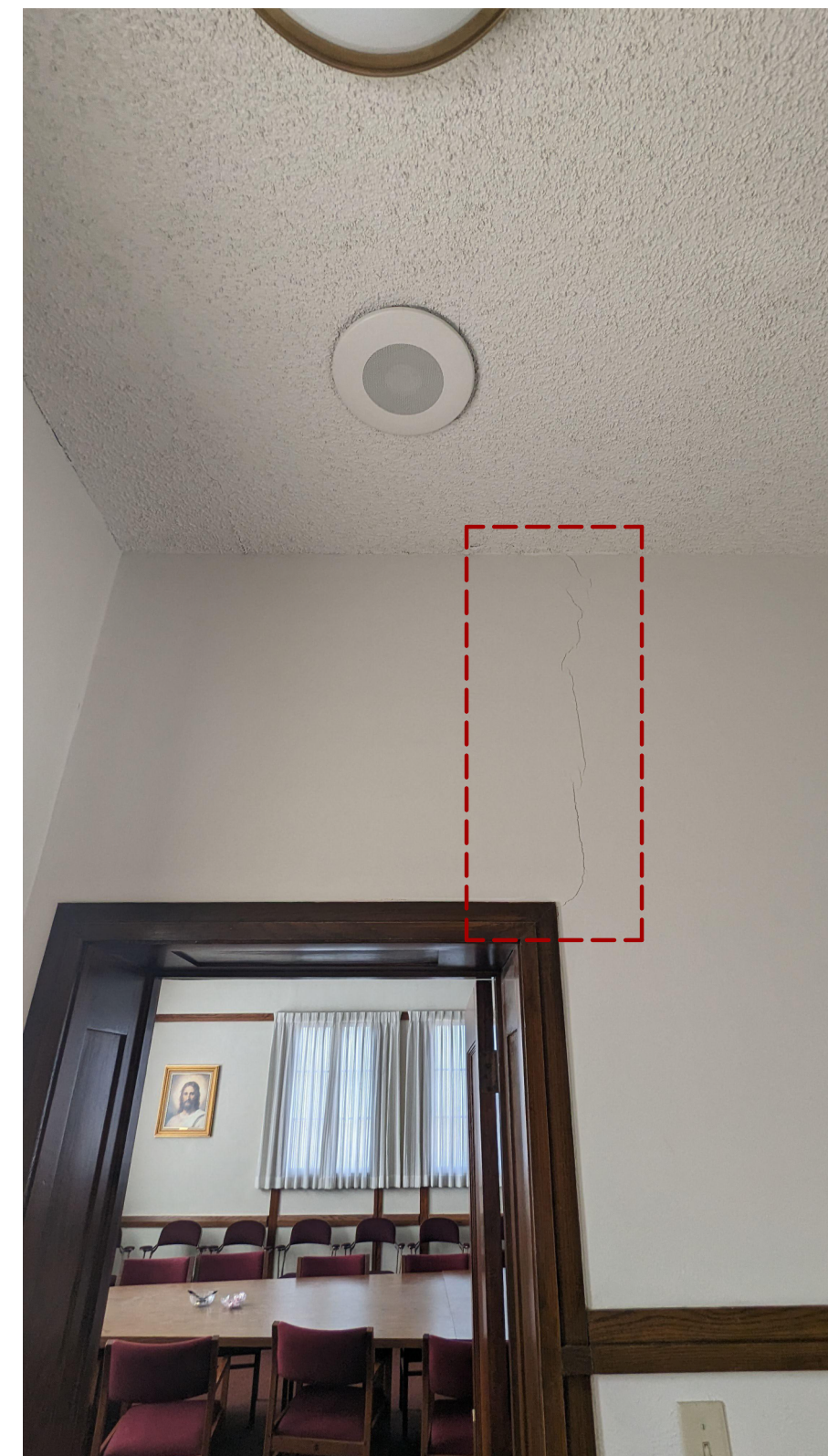
A3 CRACK AT STAIR DOOR NTS
