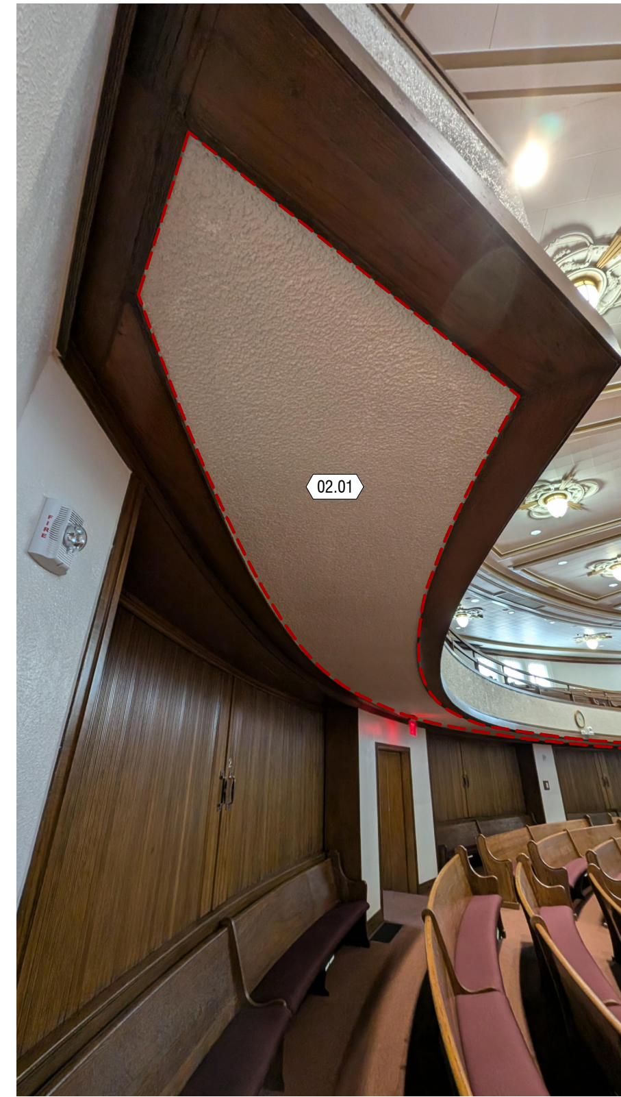
C3 ASBESTOS AT BALCONY BOTTOM NTS
